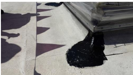
SEAL LEAKING CORNERS
