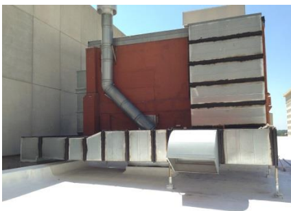
LEAKY DUCTWORK SEALING
