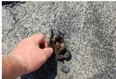
REPAIR EXISTING VOIDS
